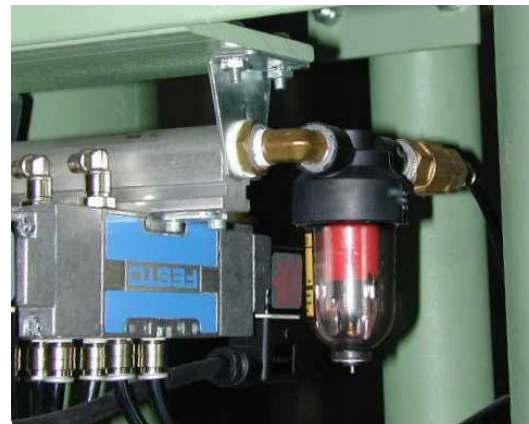
Figure 3 – Pilot Air Filter
