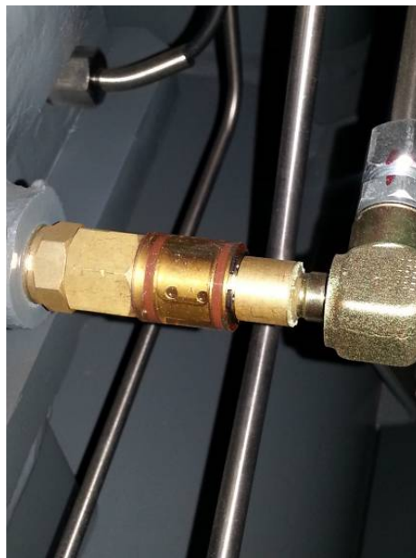
Figure 4. Scavenging Line Sight Glass.
